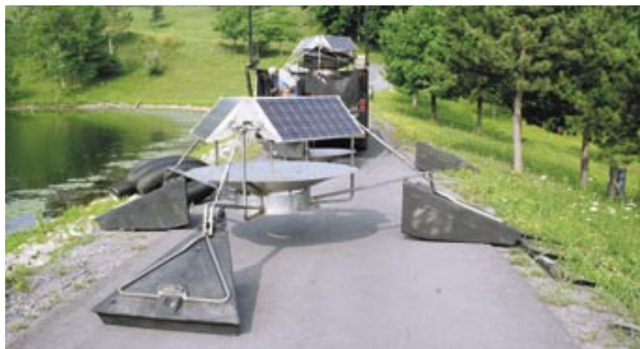
Solarbee, Inc. provides installation of their units. This one is being assembled on site, almost ready to put in the water.
