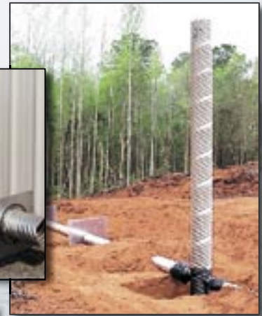
Riser T with Trash Rack
