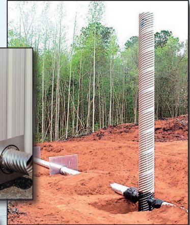
Riser T with Trash Rack
