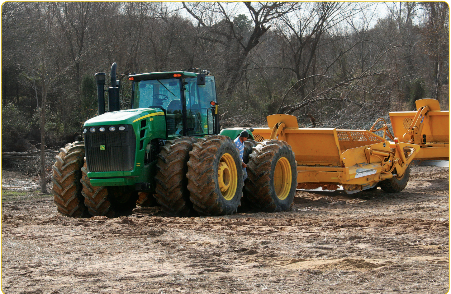
Look beneath the wheels of this heavy piece of equipment. The dirt isn't moving. It's tightly compacted.
