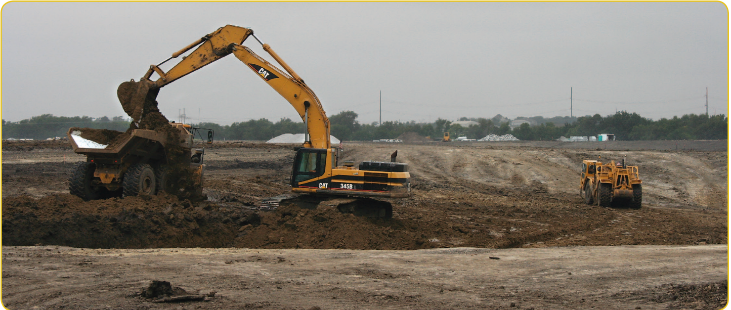
In the background, a scraper rolls over and over clay soils to compact. In the foreground, topsoil is being removed for later use. Topsoil is not good material to place in a dam. It's good for the top of the dam, to grow grass.
