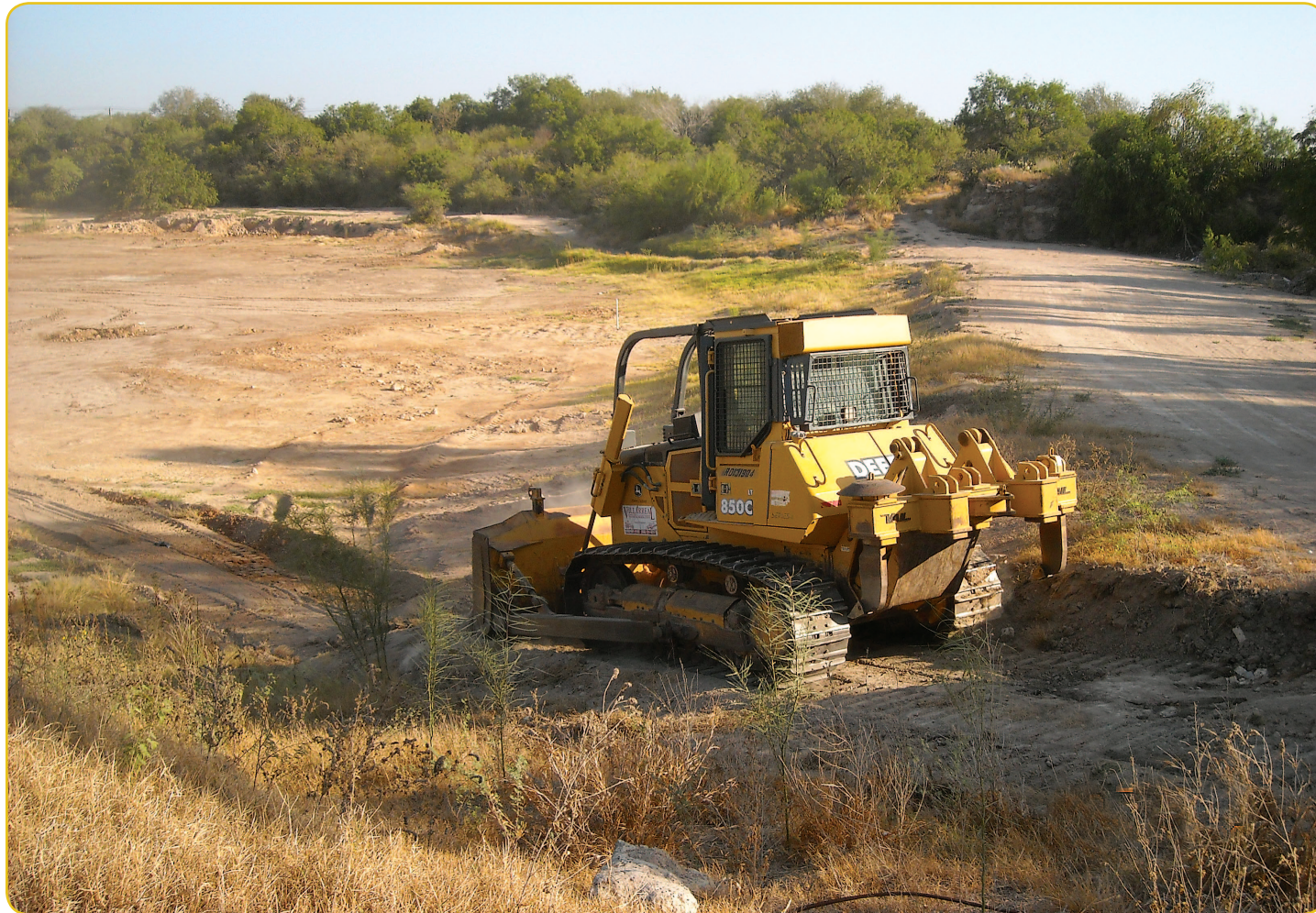
A bulldozer, although heavy, isn't as efficient in compacting soil as rubber-tired equipment or a sheepsfoot roller. A bulldozer is most efficient pushing dirt 100 feet or less.
