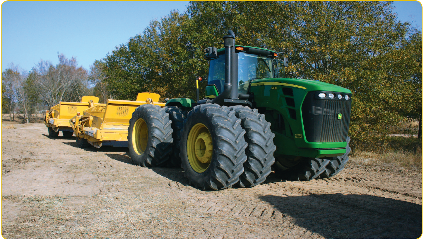
This double pan scraper is efficient in moving dirt a long distance, plus it has an added benefit. Look at the spacing of the tires, front to back. With the added weight of a load of dirt, this machine is excellent for compaction.
