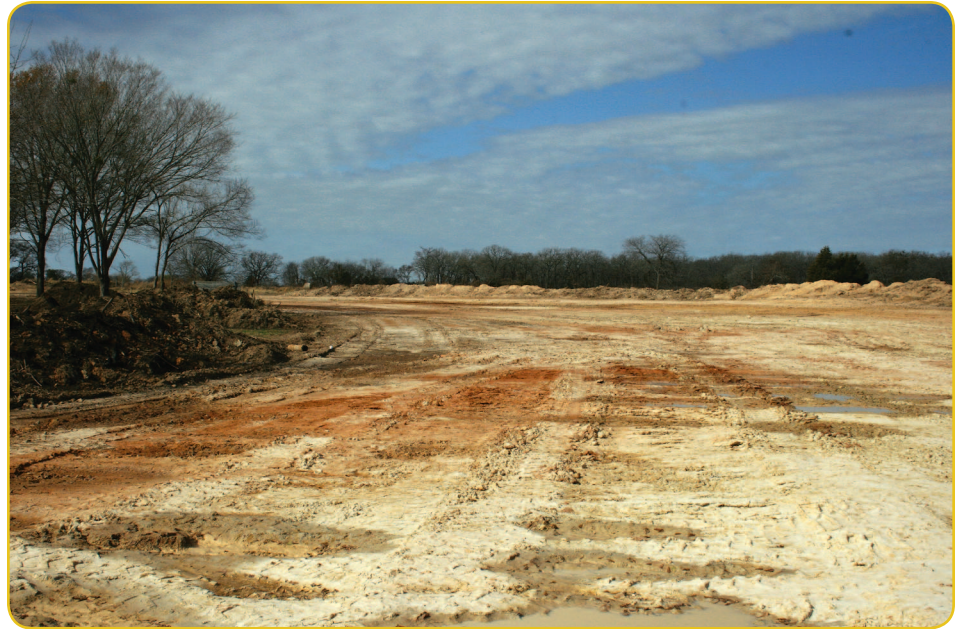
This picture shows a core trench for a fairly large dam, tightly compacted and ready for the dam to be built upward.
