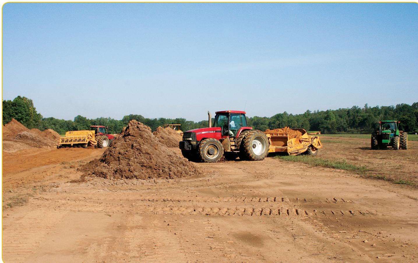
Efficiency in action. Moving lots of dirt, good lifts and great compaction.
